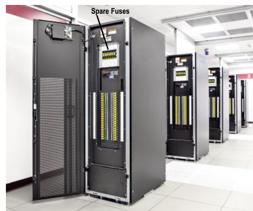
Figure 11. Remote power panel incorporating chassis QSCP with CCPB/CUBEFuse as well as spare CUBEFuses in holders. Courtesy Liebert® FDC™ power distribution cabinet from Emerson Network Power™.
