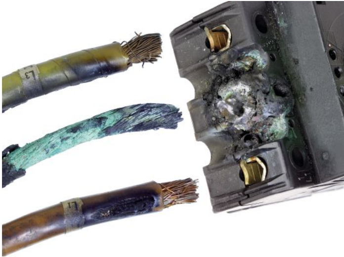
The middle, lineside conductor to this disconnect became loose. The loose connection created an excessive thermal condition that caused excessive damage to the device termination, the middle conductor and the adjacent conductors.
