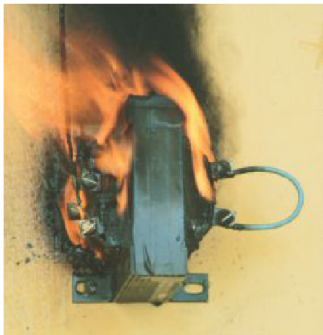
This photograph vividly illustrates the effects of overcurrents on electrical components when protective devices are not sized to the amp rating of the component.
