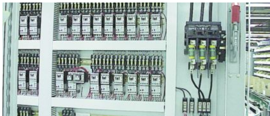
Interior of modern industrial machinery panel.
