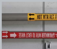
Pipe & Valve ID
