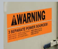
Equipment & Panel Labeling
