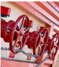
Fire & Life Safety Equipment
