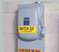
Panel & Enclosure ID
